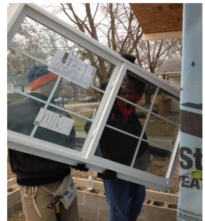
Attorneys Harold Adams (top photo) and Forrest Heyman (bottom photo) work to install windows at the build site.
